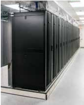
40' long Isolated Platform houses two banks of servers and IT equipment.
