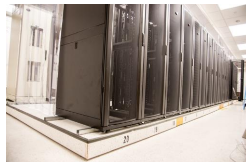
Figure 19: Isolated Platforms in the SLC PSB server room
