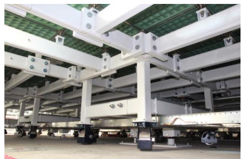
Figure 18: A 1200mm tall isolated floor system that protects two Super Computers.
