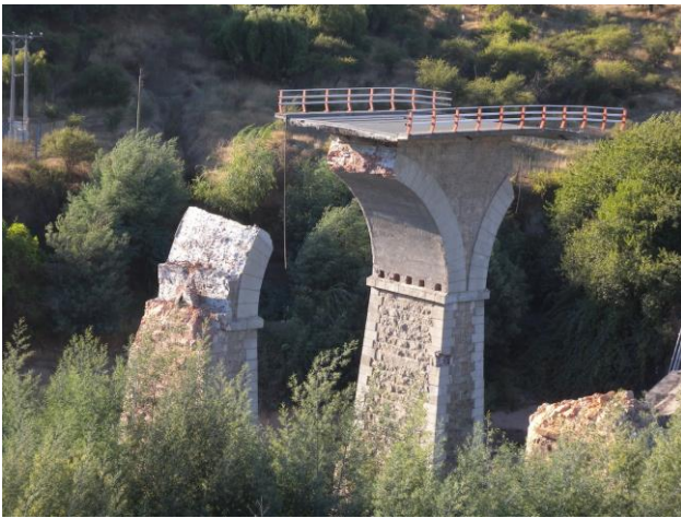
Figure 02: Destroyed Rio Claro Bridge, Chile
