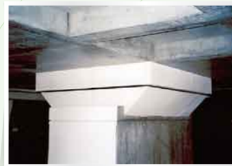
Fire board protects this isolator under the Kamikuzawa Condominiums.
