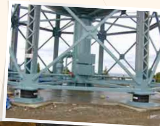
Retrofitted water tank in Seattle, Washington.
