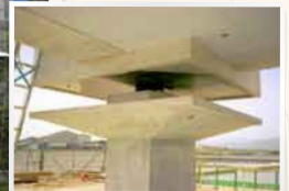
Top: Yuzawa Hospital, Japan. Bottom: A slider installed at Takasu Hospital, Japan.
