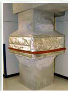
Fire blankets were used in Channing House.
